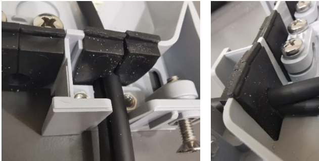
Image 5 – Cables placed in Rubber Grommet
