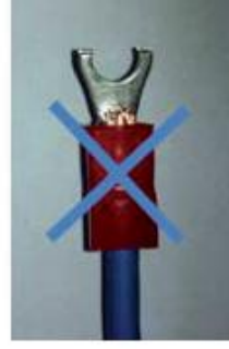
Terminal has been cut.
