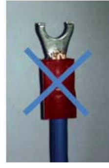
Terminal has been cut.
