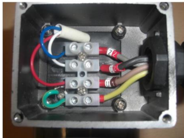
Motor Terminal Box
