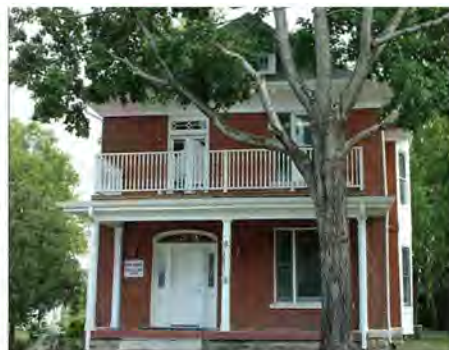
This is an older image of the Boyd House. It is in current need of major repair and has sustained significant damage to the exterior.
