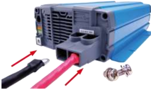
Figure 17. DC cable connection
