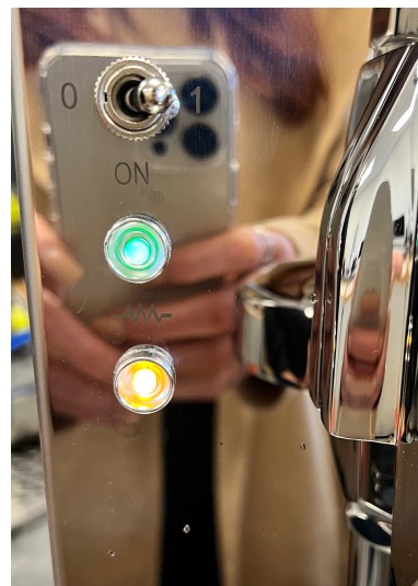
New Indicator lights & on/off switch (2021)
