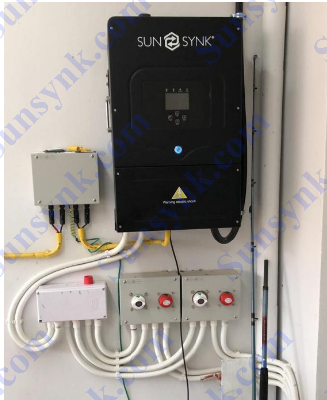
Figure 14 - Sunsynk inverter installation - black version.
