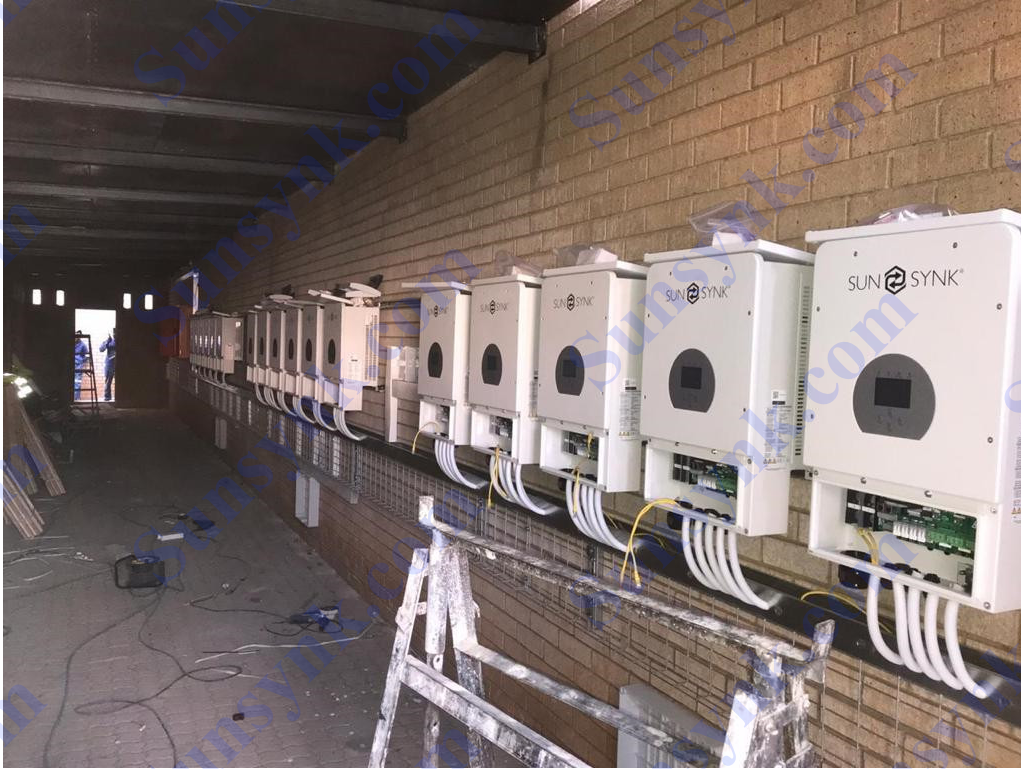
Figure 51 - Installation with many inverters.
