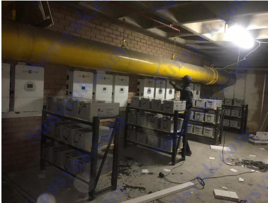
Figure 59 - Inverter installed in a dusty environment.
