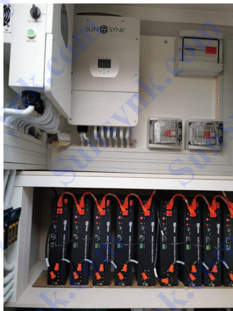
Figure 16 - Inverters with appropriate battery connections.
