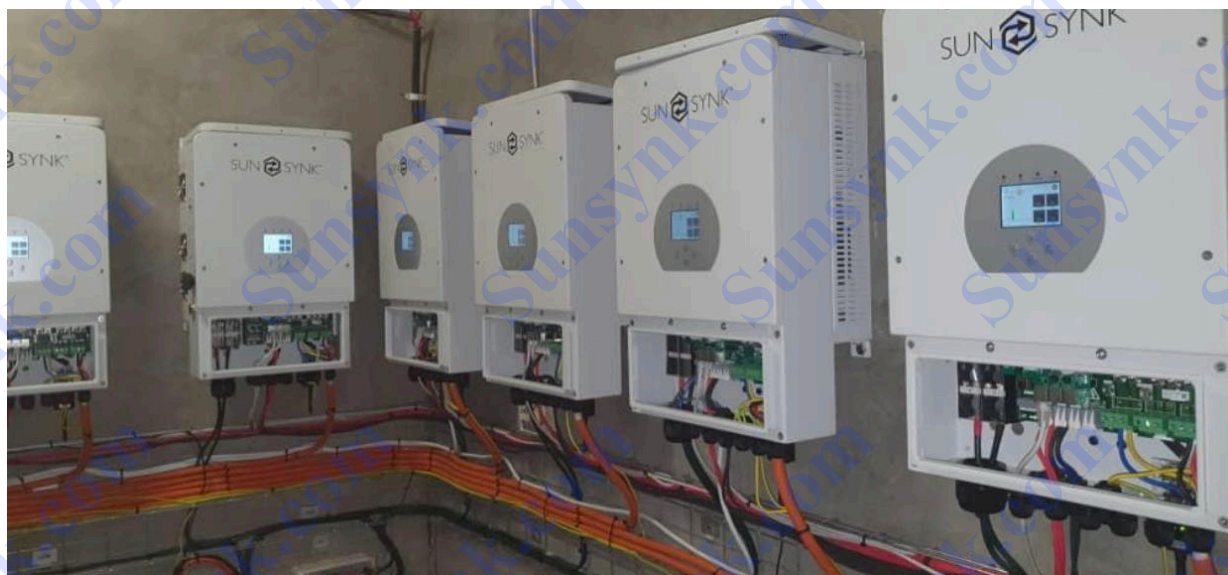
Figure 55 - Sunsynk inverters paralleled.
