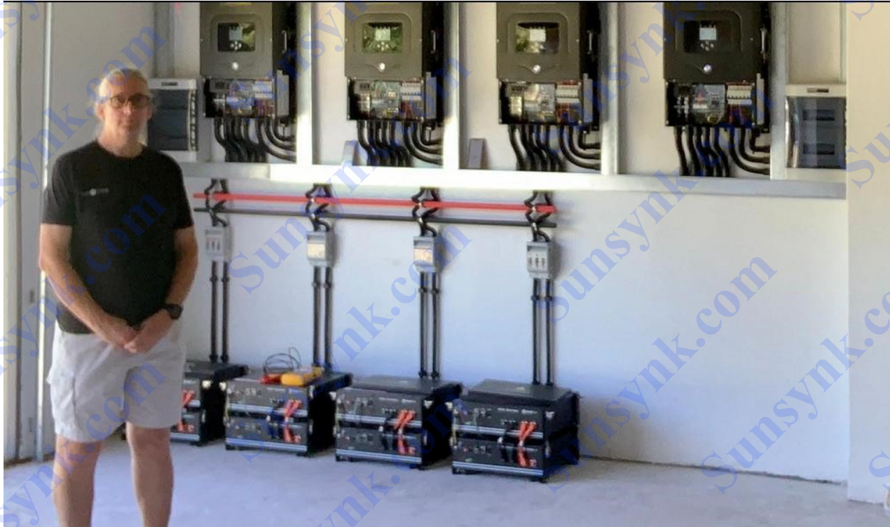
Figure 12 – Keith Gough at a Sunsynk installation in Port Elizabeth.
