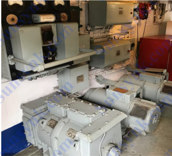
Figure 10 - Ship rotary inverter.
