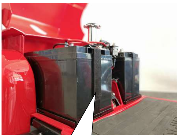
Battery tie down straps
