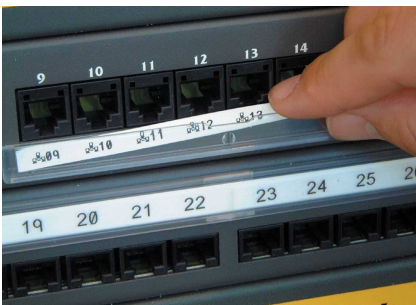
Punch block & patch panel labels
