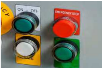
Control panel labels
