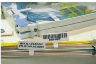
Fibre optic cable markers
