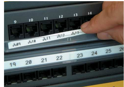
Punch block & patch panel labels
