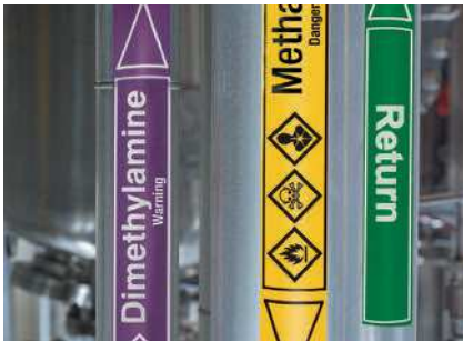
Pipe & valve marking
