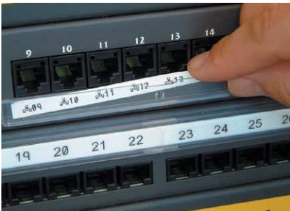
Punch block & patch panel labels
