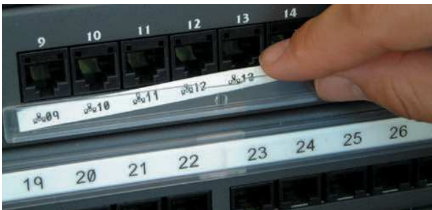
Punch block & patch panel labels
