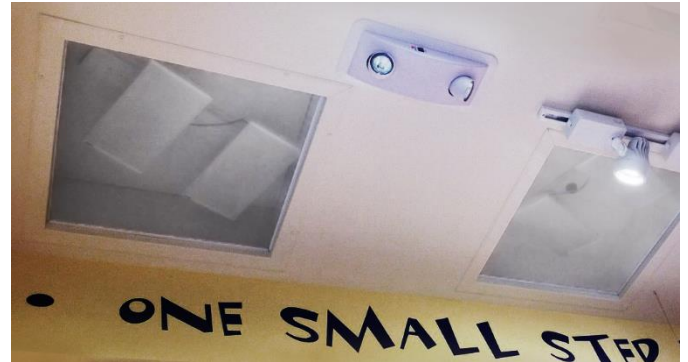
Ceiling-mounted directional audio speakers beam sound to interactive workstations throughout a Build-a-Bear Workshop.
