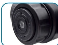
Sight Glass Window to Confirm Operation
