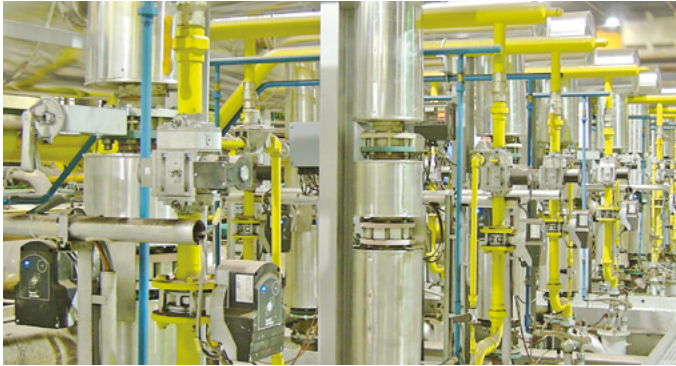
Walking beam furnace with overhead firing
