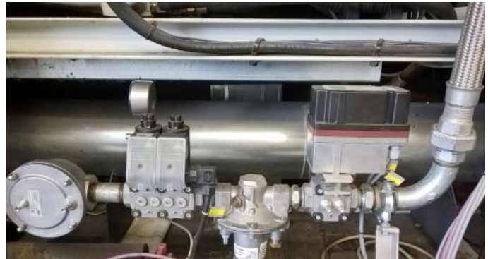
CHP for generating electricity and heat
