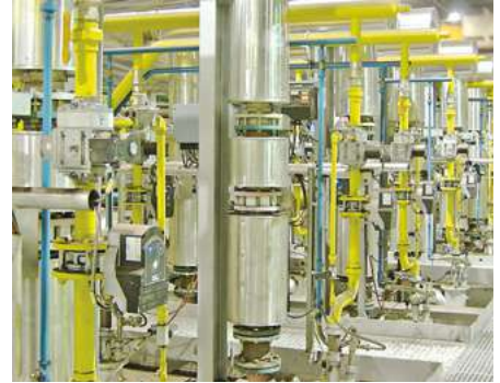
Walking beam furnace with overhead firing
