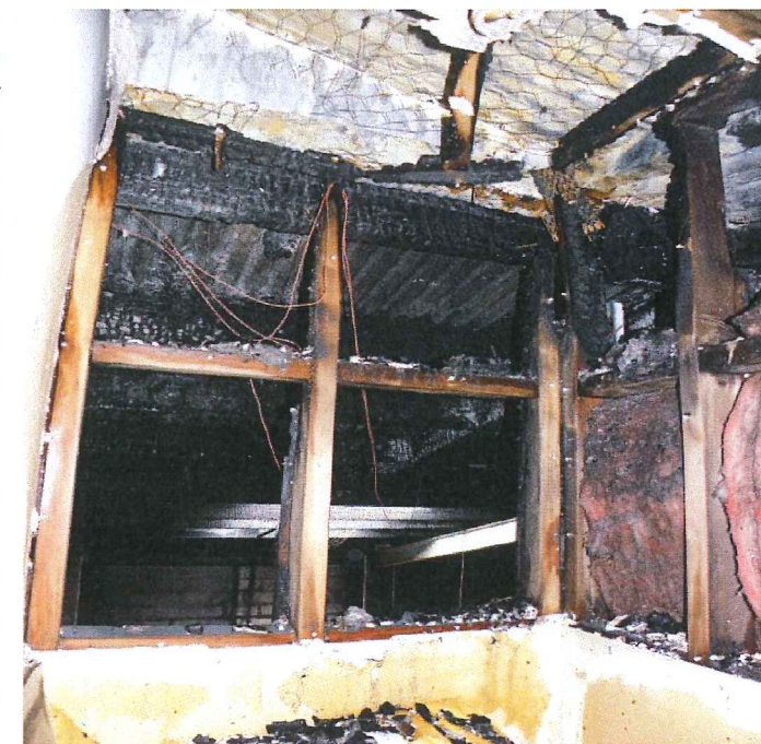
Figure 2 - First Incident: remnants of the wall separating the kitchen of the residential unit from the workshop
