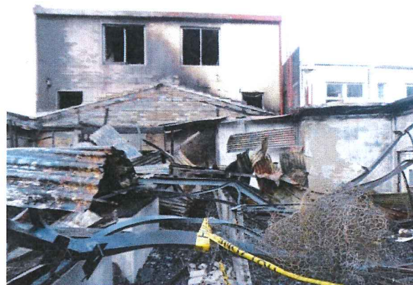
Figure 1 - Second Incident: Rear facade of commercial unit overlooking the burnt out workshop
