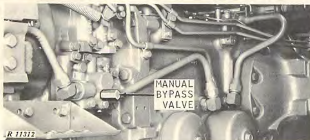
Manual Bypass Valve on a Power Shift Tractor
