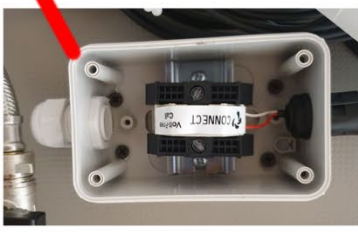
Voit Free Coil Heating controls
