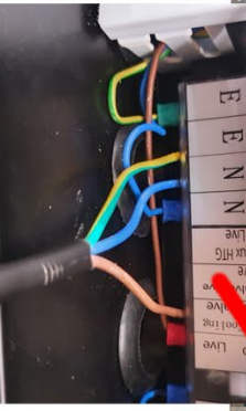
Heat Pump HW Valve Live 3-Port Valve Connection
