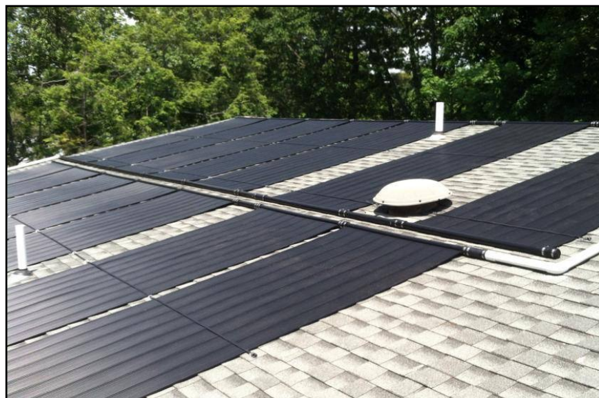
Using various configurations of hoses and header spacers, this system avoids roof obstructions while maximizing the solar collector area. (Photo courtesy of Solar Living - Fair Lawn, NJ)
