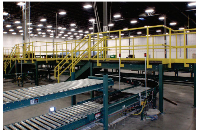
Conveyor Crossover Integrated into Existing Conveyor Operations
