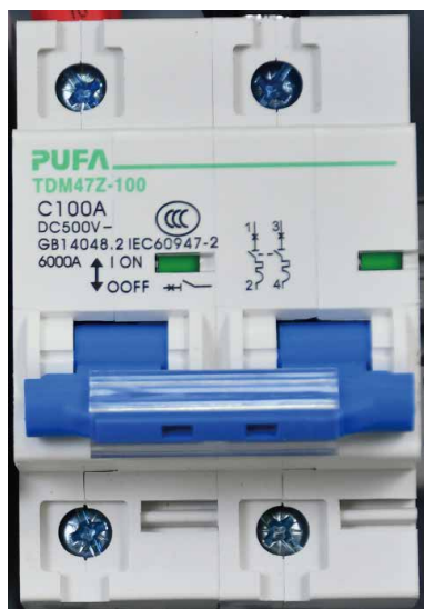
Circuit Breaker OFF
