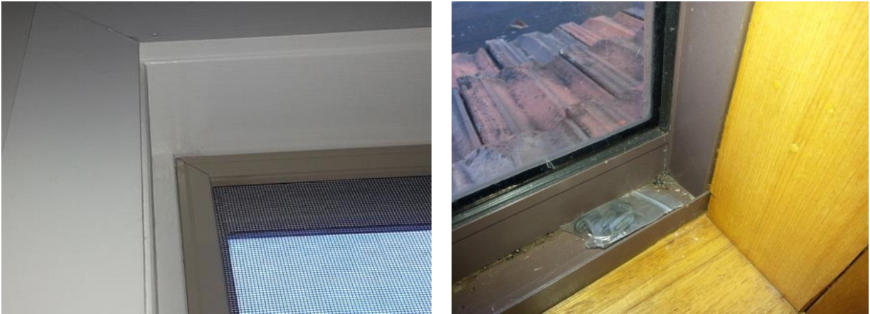
FIGURE 16: EXAMPLES OF WINDOWS WHERE THERE IS INSUFFICIENT SPACE TO INSTALL WINDOW FILM
