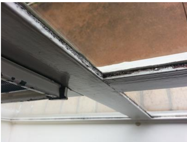
Rough paintwork on wooden frame window
