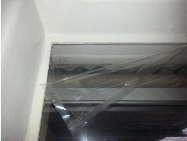
Rough paintwork on metal frame window
