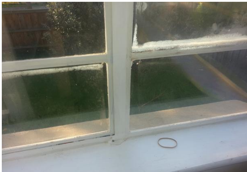
FIGURE 19: CONDENSATION TRAPPED BETWEEN THE ORIGINAL PANE OF GLASS AND THE WINDOW FILM
