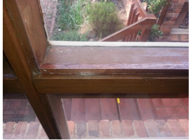
A new piece of wooden framing was installed at this property allowing for the window film to be installed.
