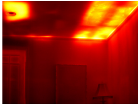
Thermal image showing clearance around downlight and missing batts.
