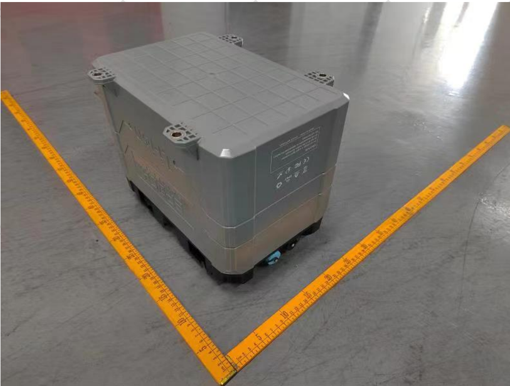
Figure 2 Overall view II of battery
