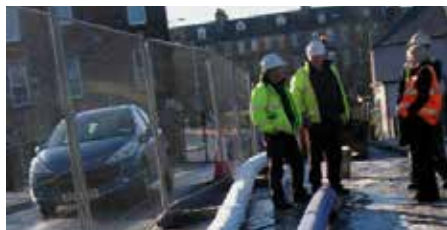
Shallow water piping process
