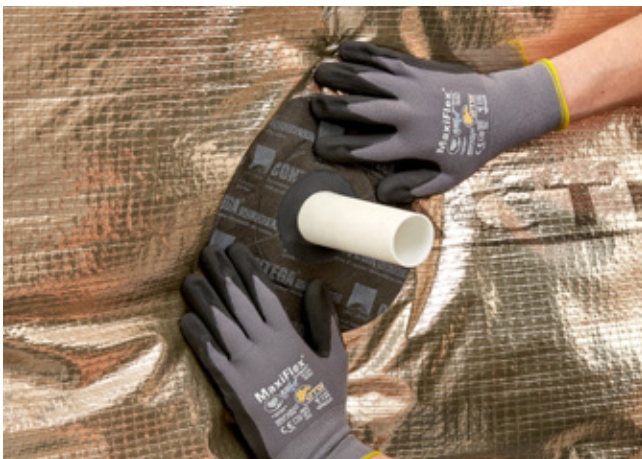
Fix grommet around pipes and ducting
