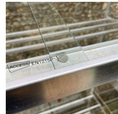
Roof glass overlapping
