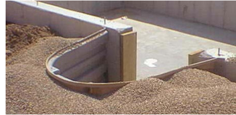
Installed Modular Well
