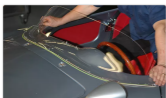
Gently pull both sides together to give the Plexi a little tension, at the same time have someone mark the locations of all the pre-drilled holes in the Plexi.
