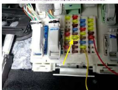
Remove the trim panel under the main driver, find the power supply, and unplug the original car 20A fuse.
