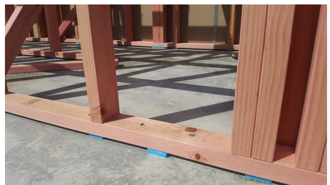
Bracing element showing additional bottom plate fixings and suggested additional packer on concrete floors.
