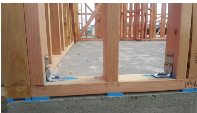
Bracing element showing “Proprietary” hold down bolt/bracket.
