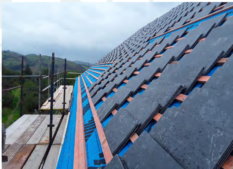
Use of chalk line to mark, perpends, half bond and slate head-line.
