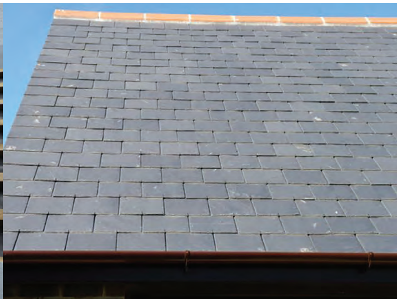
The result of installing slates without prior grading, slates of varying thickness in the same course, an unsightly, "gappy" roof slope!
