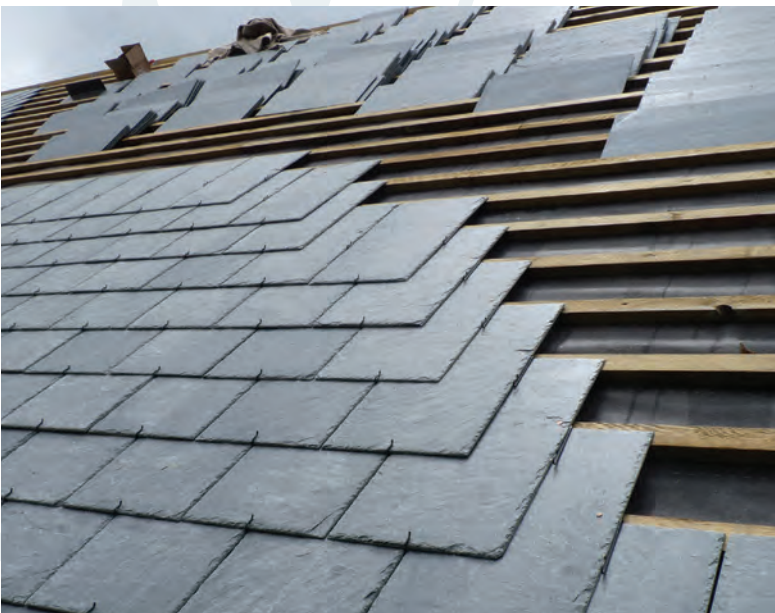
Slates graded and sorted into batches of equal thickness prior to installation
