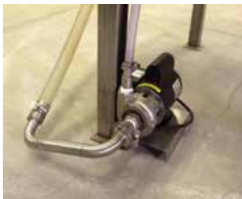
¼ HP Wash Pump
