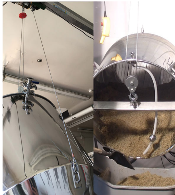
Figure 12: Mash Colander tipping cable
