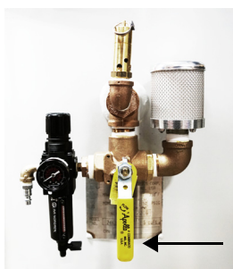
Ball valve in the closed position
