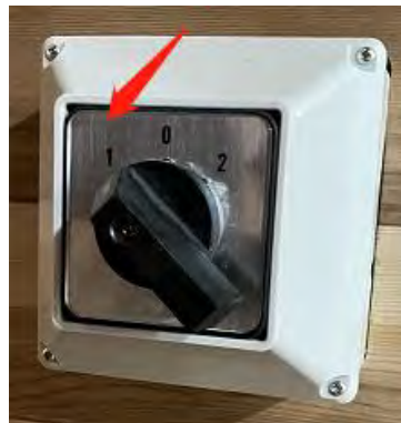
Power to stove heater
