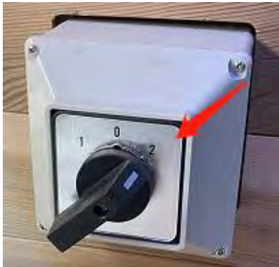
Power to Infrared heaters
