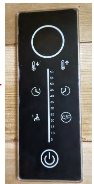
Sauna Control Panel has no Illumination
