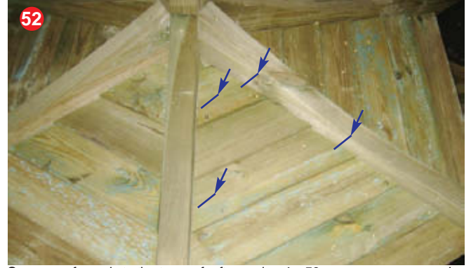
52 Secure roof panels to the top roof rafters using 4 x 50mm screws per panel.
