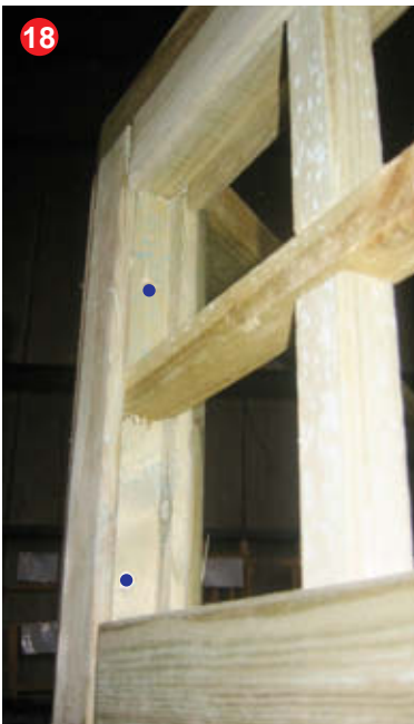
Secure fence with 4 x 50mm screws, 2 at each end of the fence.
