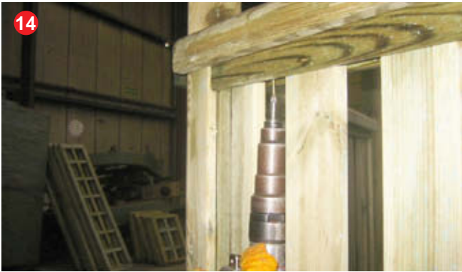
Secure hand rails by screwing through fence into handrail using 3 x 40mm screws.
