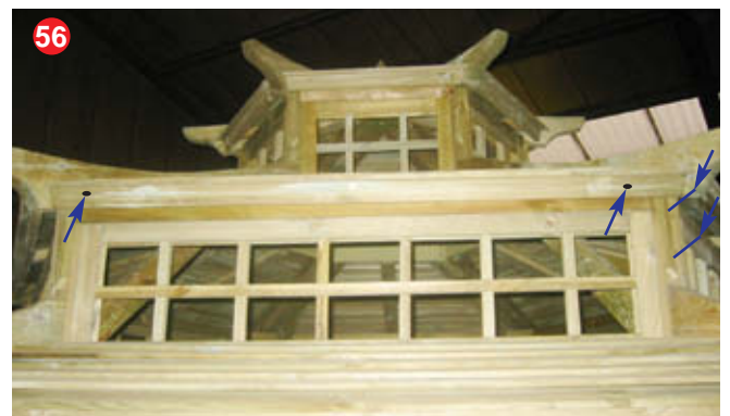
56 Fit 6 roof panel fascia boards and the 6 finials using 2 x 50mm screws each.
