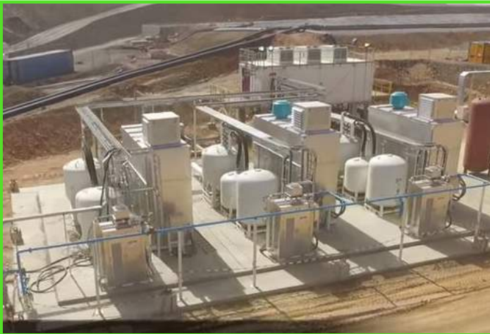
Mining Processing Application, Redundant DOCS 500
