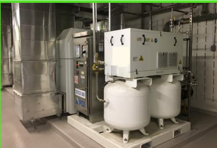
Water Treatment Application, Redundant DOCS 500
