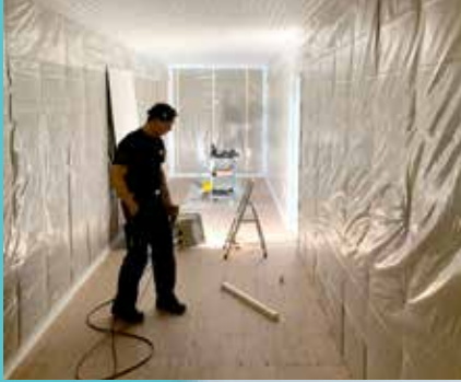
The containers are insulated.
