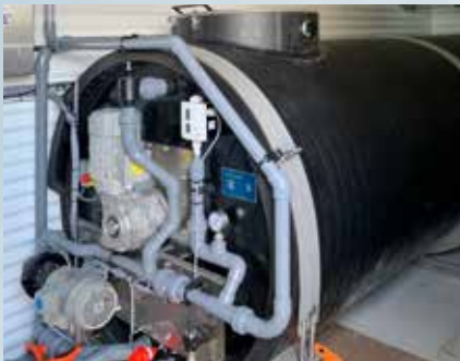
Storage tank for the liquid ice to control better the cooling of the product.
