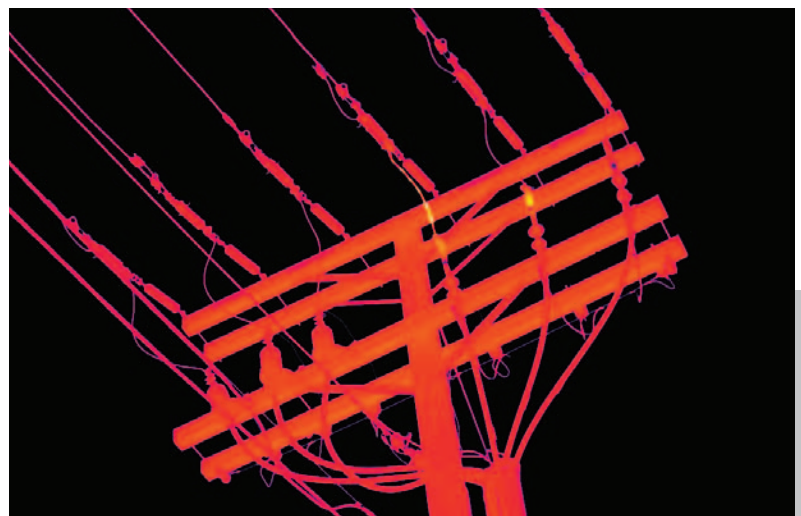
Electrical utility distribution lines
