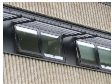
External shading (brise soleil) to mitigate summertime peak solar gains
