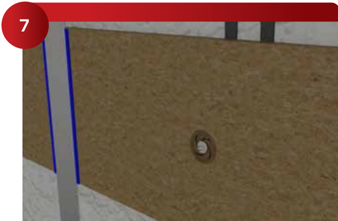
Install the 224 Galaxy using a Dead-Blow Hammer. The 224 Galaxy is flush with the panel surface.
