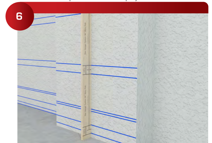
6 Layout a story pole that includes the benchmark, top and bottom of the Bars and Clips, they are 3" apart. The bars should be about 24" apart. Proceed around the space marking at the bottom of the clips at every stud.
