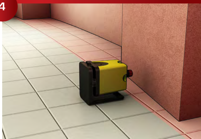
Determine greatest projection (bump out in wall). This will determine the face of the panels. Discuss the layout options with the GC. If there is a large bump you have two options, shim out most of your furring or have the projection corrected.
