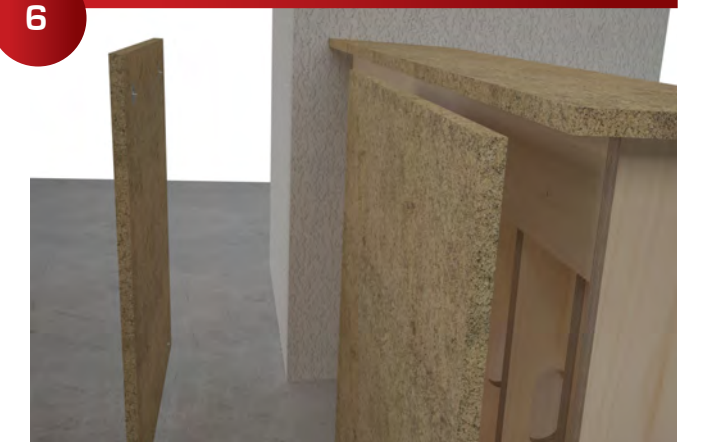
Carefully place the panel in the correct position and bump the panel in each corner to mark the location of each mounting screw.
