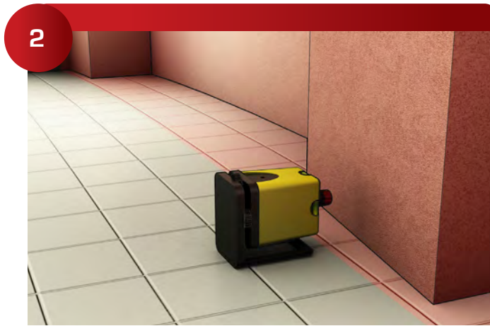
Determine greatest projection (bump out in wall) to determine face of panels on a floor layout. (Working Plane)
