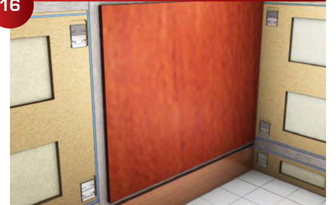
Lift the panel into place about 1/2" above marks, push in and down firmly to lock the panels into their final position.
