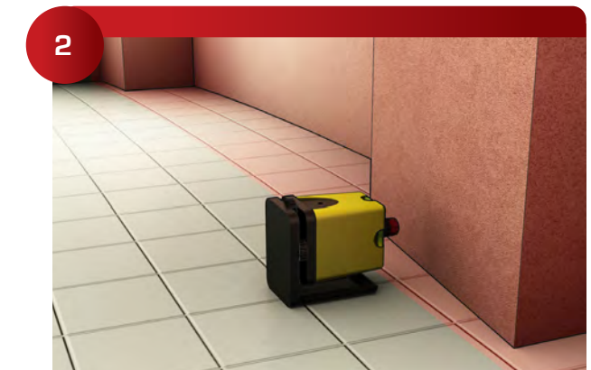
Determine greatest projection (bump out in wall) to determine face of panels on a floor layout. (Working Plane)
