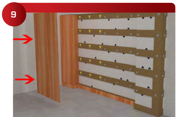
9 Place reveal spacers between panels to locate the exact panel positions. Carefully push the panel into the 410 NZ Alignment Clips to mark the panel clip position.
