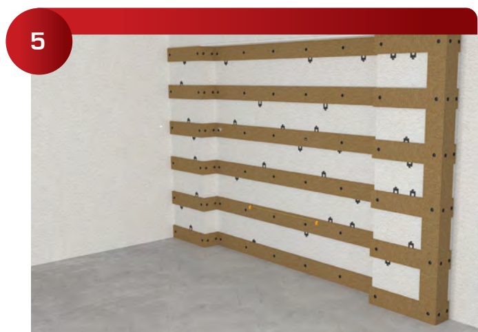
Using string lines or a laser, shim, glue, and screw all horizontal furring into place.
