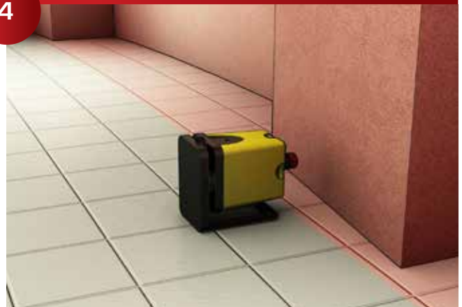
Determine greatest projection (bump out in wall). This will determine the face of the panels. Discuss the layout options with the GC. If there is a large bump you have two options, shim out most of your furring or have the projection corrected.
