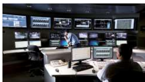
Command and control center
